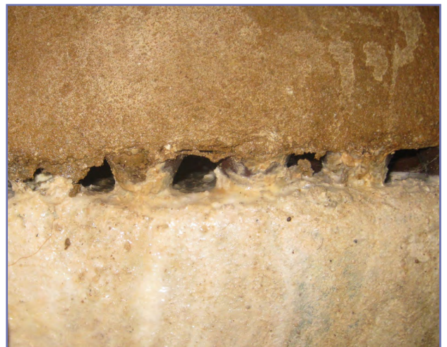
Figure 1: When free lime completely blocks a Type C system, leading to total system failure
